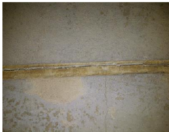
Photo #10- cohesive failure
