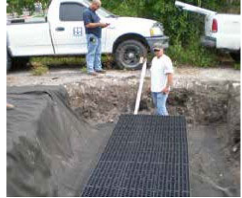
R-Tank LD Field Testing
