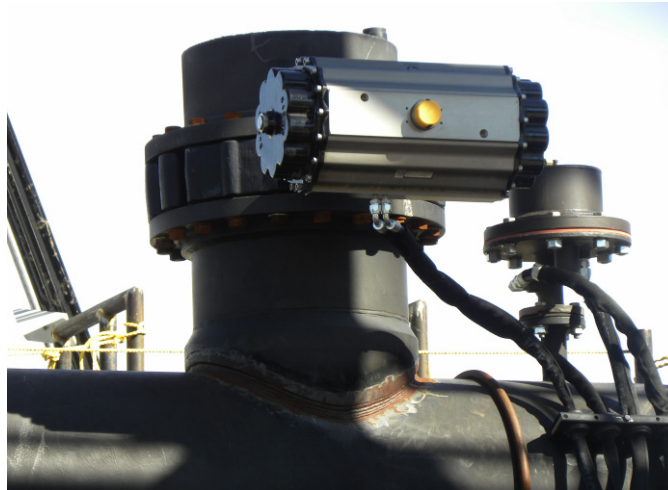
Figure 6. Slurry dilution valve with vacuum transmitter.
